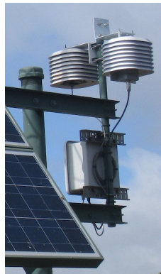
Meteorological Sensors (pressure, temperature)
