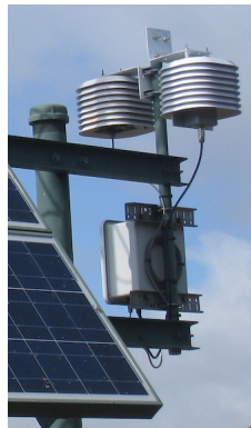
Meteorological Sensors (pressure, temperature)
