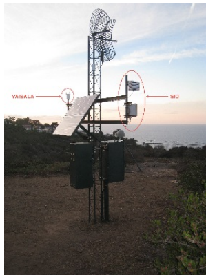
Meteorological Sensors (pressure, temperature)
